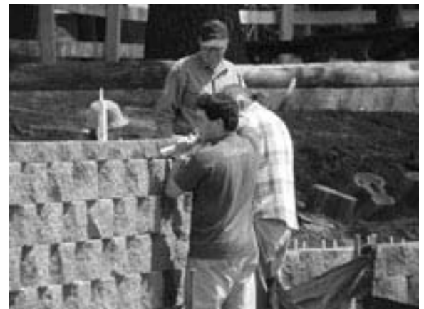
Service at Work: Jim Keene (rear) supervises the work to complete the new waterfront retaining wall at Camp Hinds in 2000. His work has been instrumental in the revitalization of all council properties.
